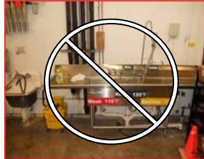
(3 compartment sink improperly installed)
